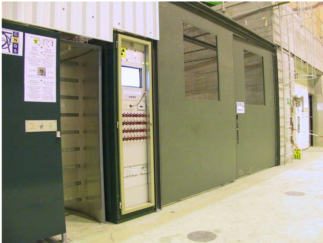
Figure 7: CNGS access point in ECA4, with material door PPG CNGS.
