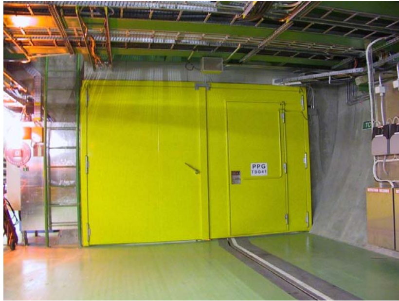
Figure 11: PPG TSG41, separating the target chamber air volume from TCV4.
