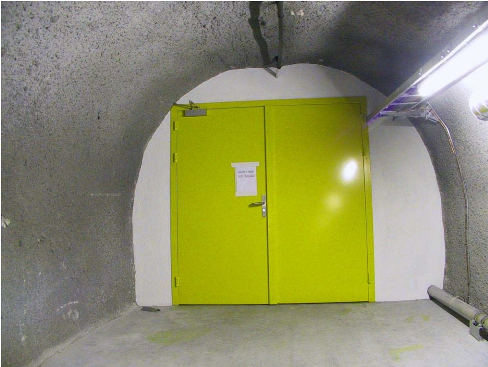
Figure 15: Ventilation and fire protection door V/F TAG42, separating TT41 from TAG42.
