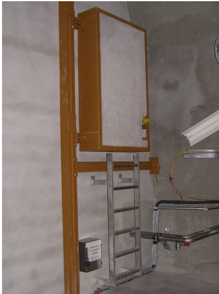
Figure 22: Shielded door separating TNM41 from the hadron stop chamber TNB4.
