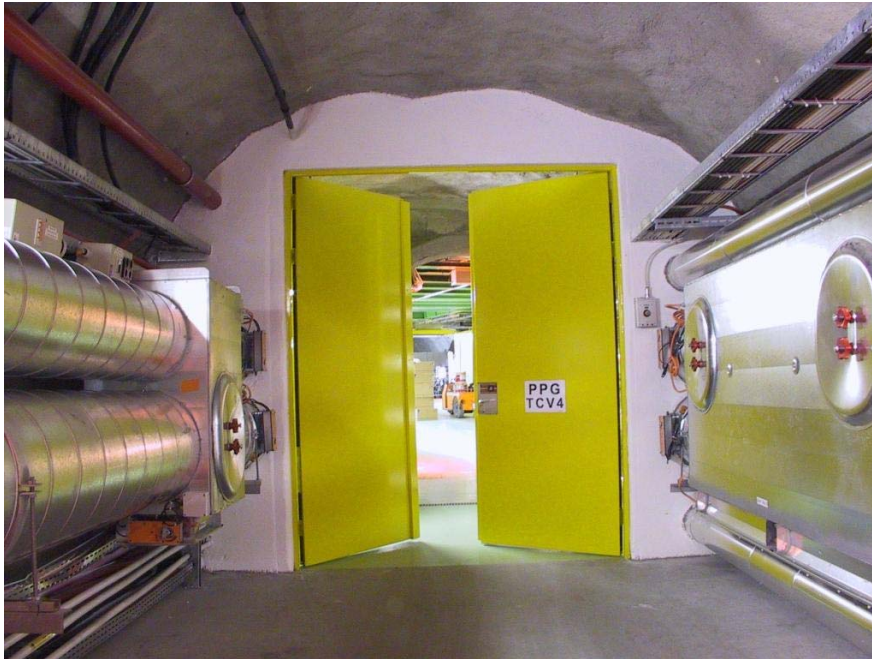
Figure 9: PPG TCV4, at the entrance to the ventilation chamber (here, both wings are open).
