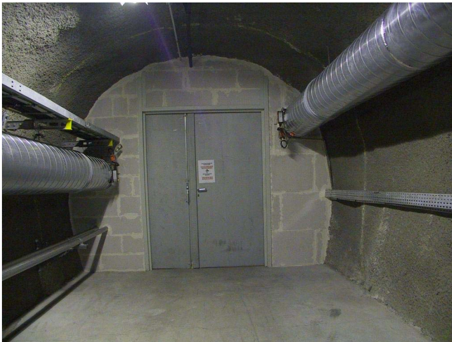
Figure 20: Ventilation and fire protection door V/F TZ80
