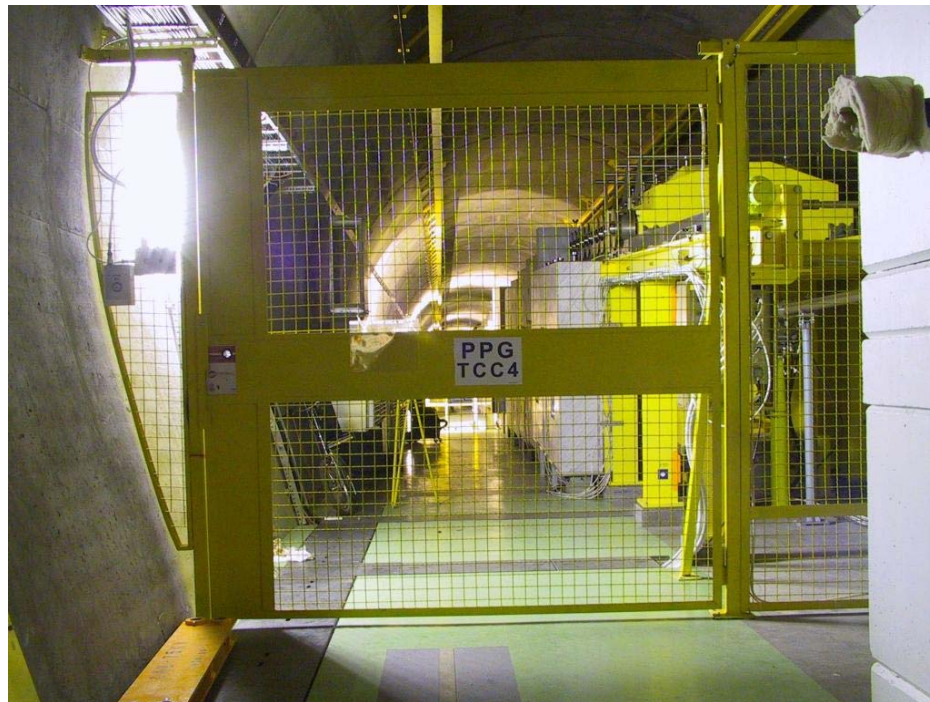
Figure 18: PPG TCC4, separating the high radiation area and the "local électrique" (open stripline connections) from the upstream part of TCC4.
