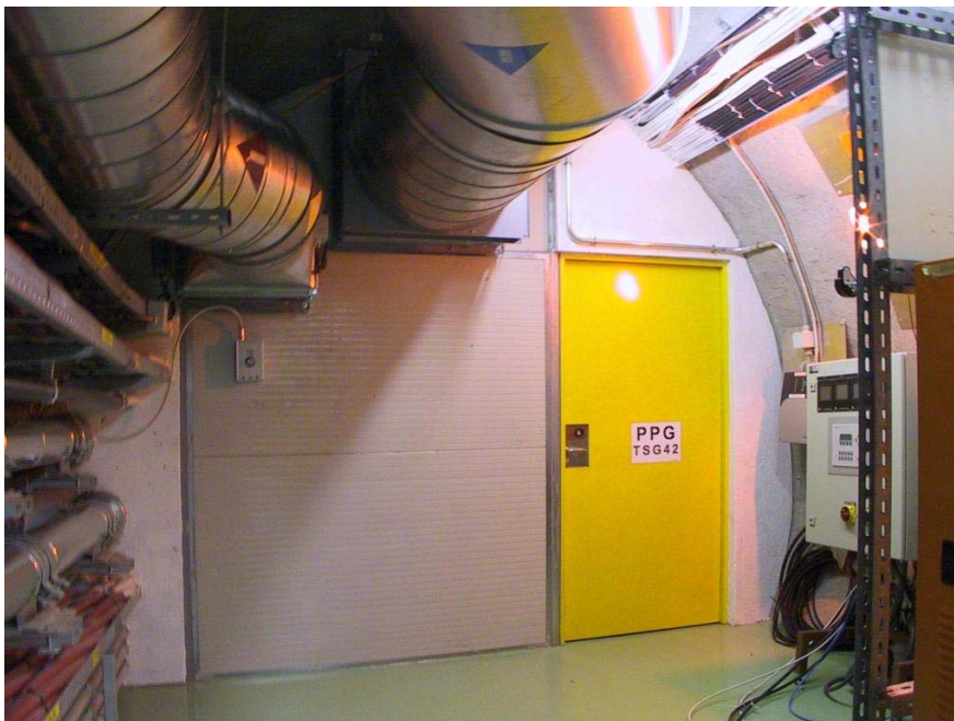
Figure 10: PPG TSG42, downstream of the electronics racks in TSG4.
