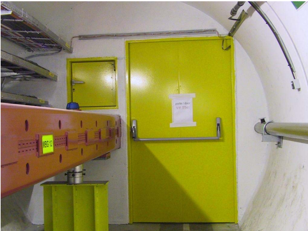
Figure 16: Ventilation and fire protection door V/F TT41, separating TJ8 from TT41.
