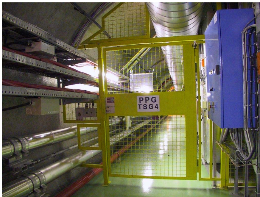
Figure 17: PPG TSG4, separating the "local électrique" from the upstream part of TSG4.
