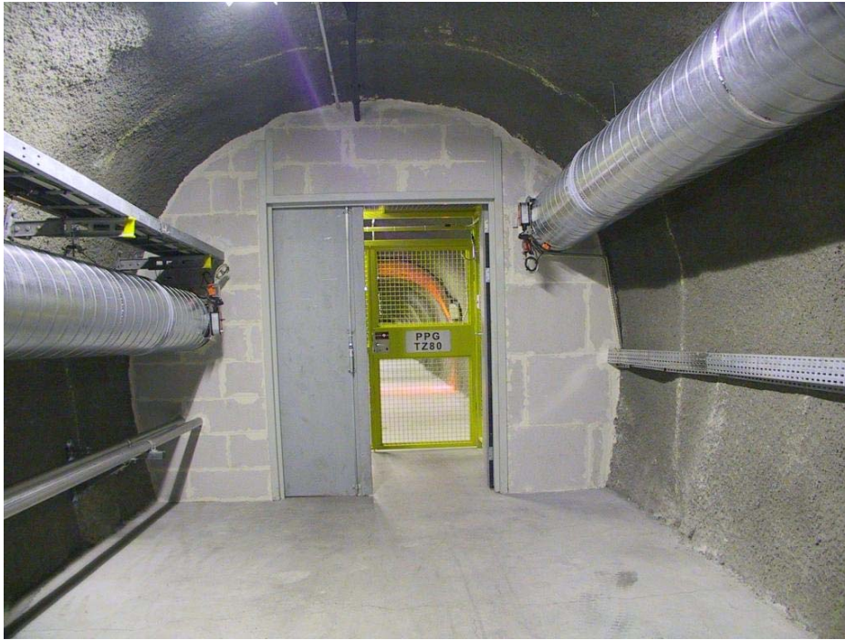
Figure 21: Access door PPG TZ80 seen through the (opened) ventilation door V/F TZ80.
